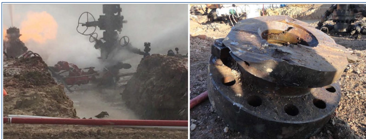
Figure 122—Jet cutting operation to cut the wellhead. The position of the jet cutter below the lower-most leak (left) and the cross section of the cut afterward (right)
